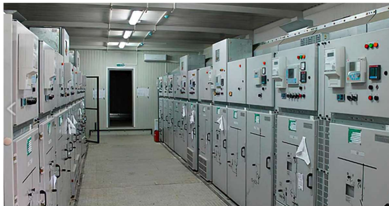
Picture 1.7 – transformer substation
