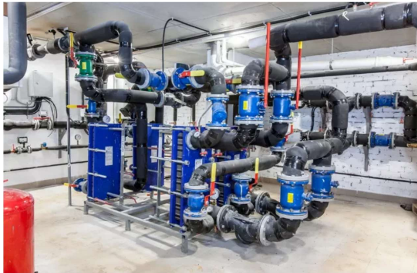
Picture 1.6 – Central heating system
